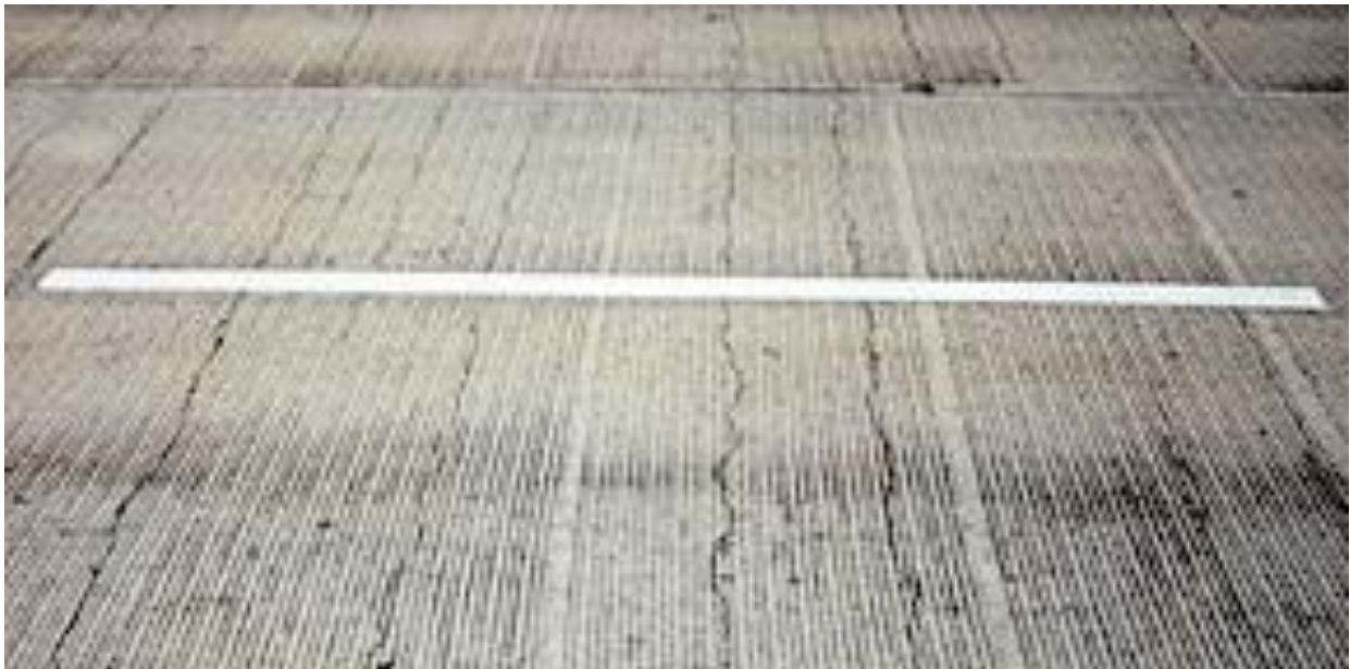
Figure 1. Early-age shrinkage cracking of a bridge deck (Kosmatka and Wilson 2011)
