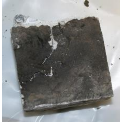
Figure 49. The black material within the crack seems to be a sealer such as linseed oil (Core C1_8407_C)
