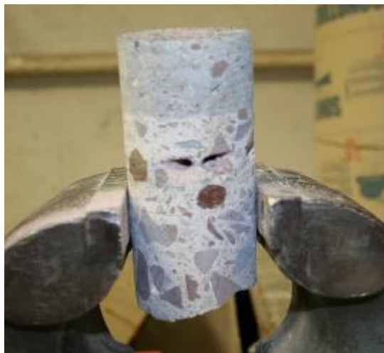
Figure 46. An example of a core with drill holes at the rebar level.
